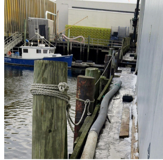
Pier with infestation
